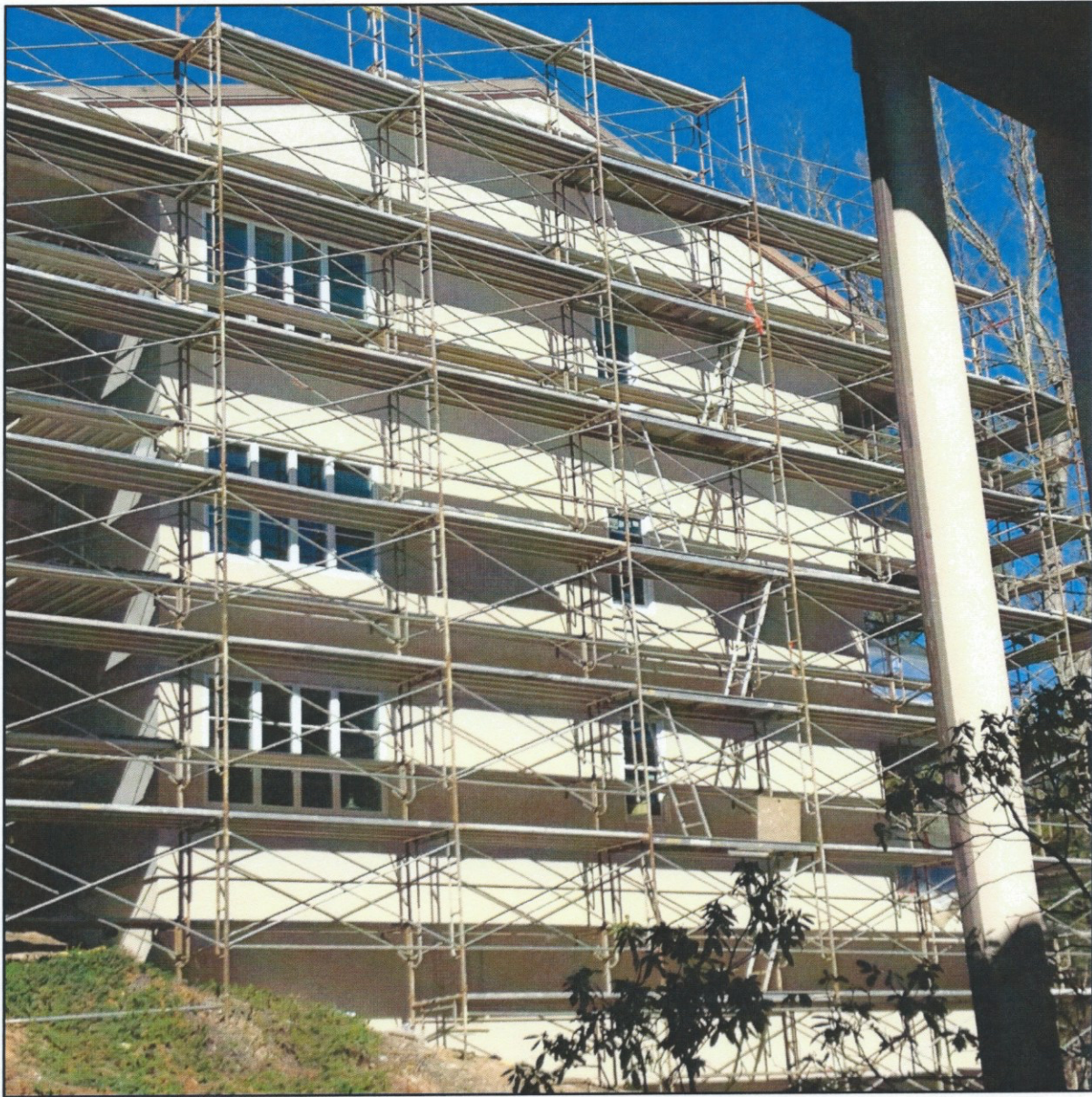
The EIFS finish coat application at the east end wall and the tall corner column is in progress.
