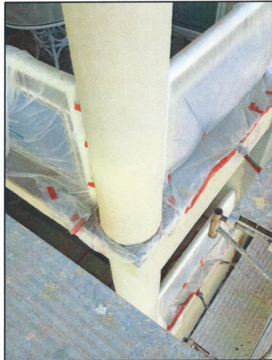
Views of rear porch column work being completed with the urethane deck coating and touch up painting.
