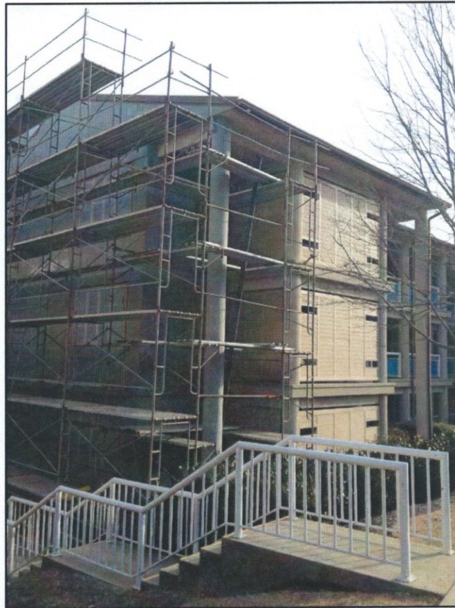
The EIFS base coat application at the west end wall and the tall corner column is in progress.
